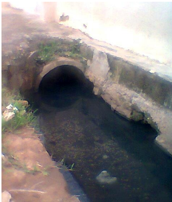
Plate 2: Torrential rain in yellow duke Road
